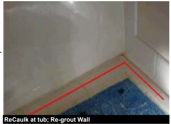
ReCaulk at tub; Re-grout Wall
