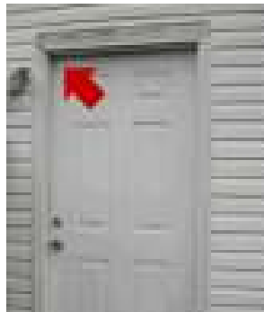
Damaged frame molding
