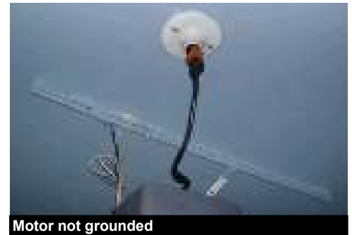
Motor not grounded
