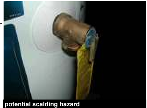
potential scalding hazard
